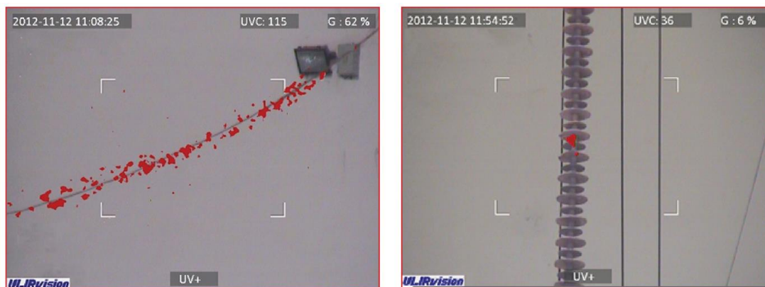
Figure 3.3. UV image of a corona discharge on a power transmission line
