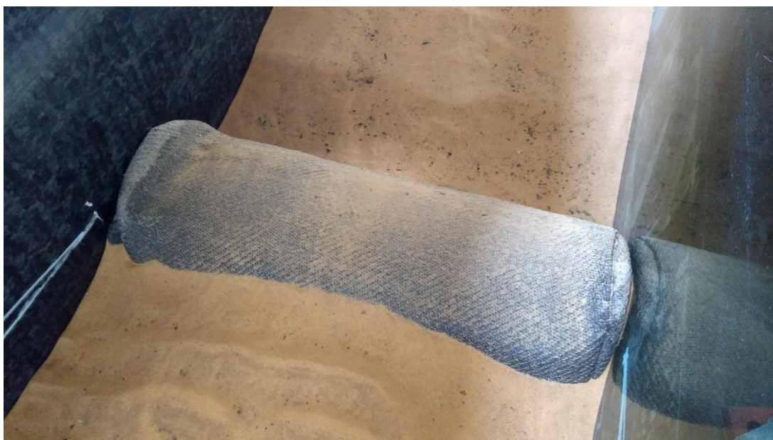
Figure A.9. Post-Storm Scour Around Geotextile Tube
