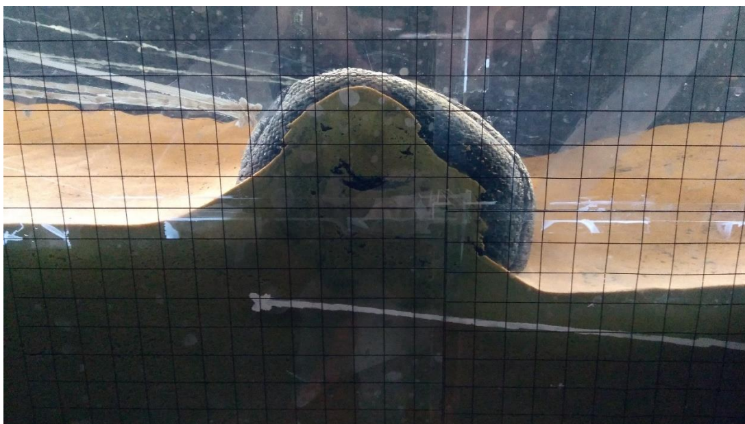
Figure A.10. Post-Storm Erosion and Scour Around Geotextile Tube
