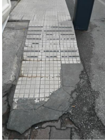
Figure 4.29. Narrow and deformed curb ramp
