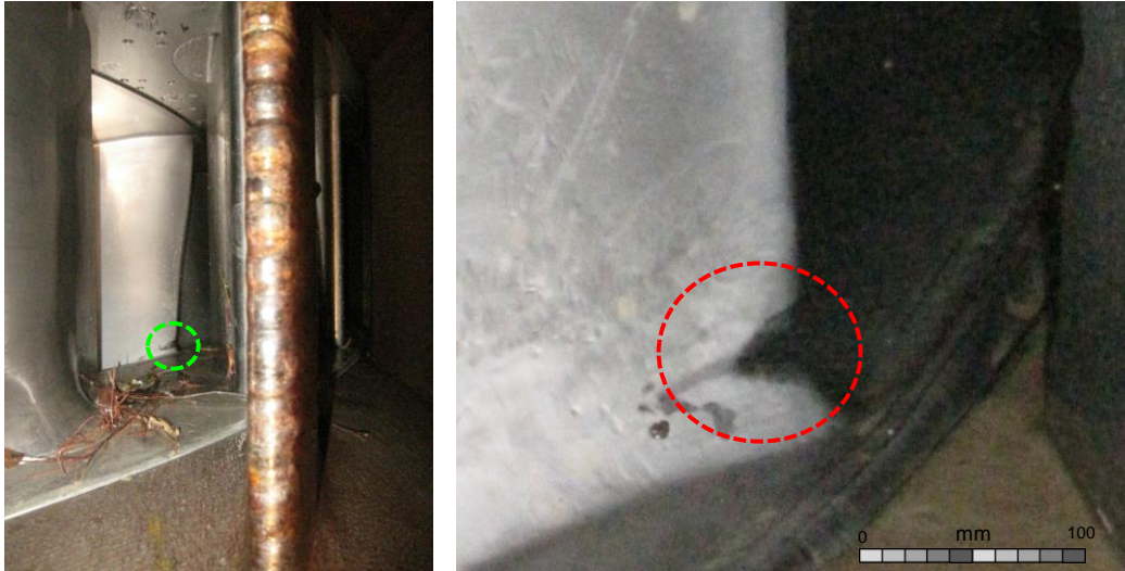
Figure 2.49 : Cracks in the runner blades, view of the pressure side
