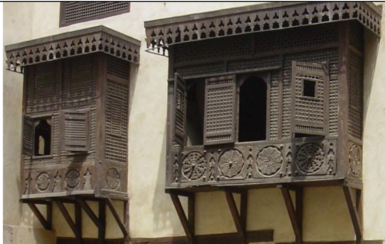
Figure 58: Mashrabia. AL- Sennary House. Egypt source: http://www.egyptarch.net/historicalcairo/islamicmonuments/senaryhouse/senary2.htm (last retrieved on 11 may 2016, at 18:00)
