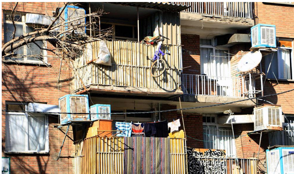
Figure 11: Misusing of Balconies in Tehran Source: http://www.zamoune.com/ (Last retrieved on 16 September 2015, at 11:00)
