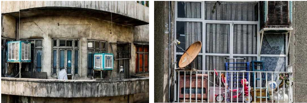
Figure 6 & 7: Misusing of Balconies in Tehran
