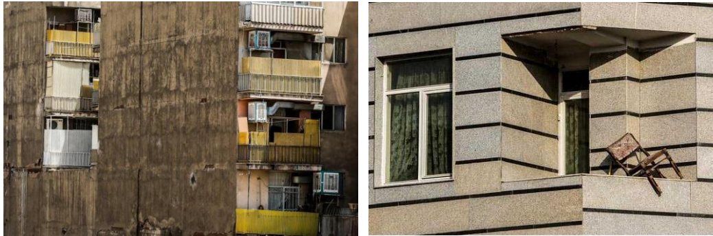
Figure 4 & 5: Misusing of Balconies in Tehran
