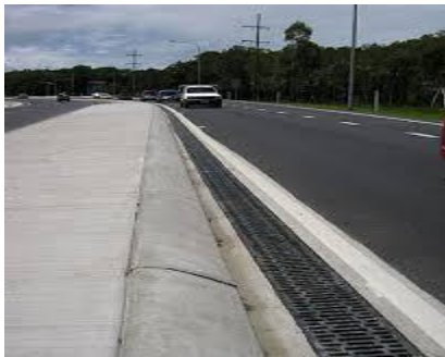
Figure 2.3 Continuous Grate Inlet in Site
