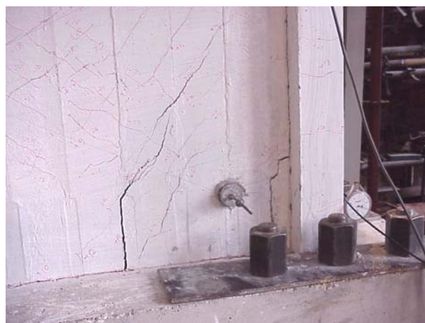
Figure 5.46 – Infill Cracking, Specimen CID4
