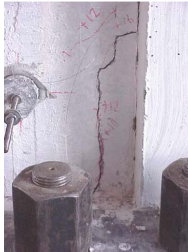
Figure 5.45 – Separation of the Column from the Infill, Specimen CID4
