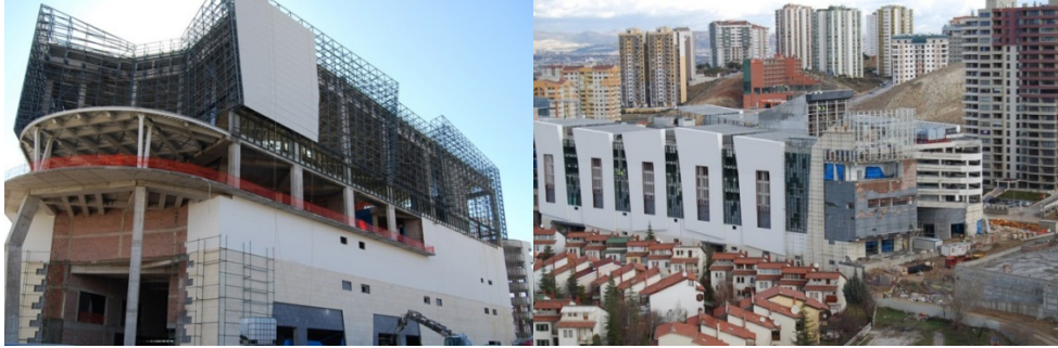
Figure 28. GORDION Shopping Center (under construction photos) – Views [Source: Gürtaş İnşaat, http://www.gurtasinsaat.com.tr/gurtas2/page_en.php?ID=131 (accessed on 21.06.2009)]
