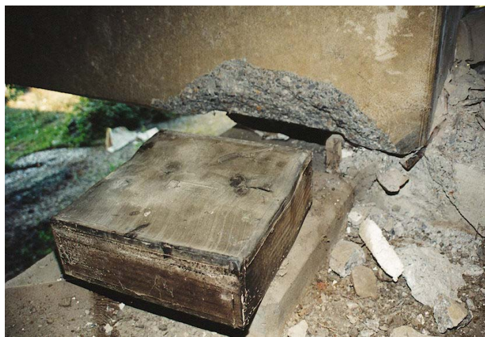
Figure 3.15 Dislodgment of bearing systems at Sakarya Viaduct (KOERI, 2009)
