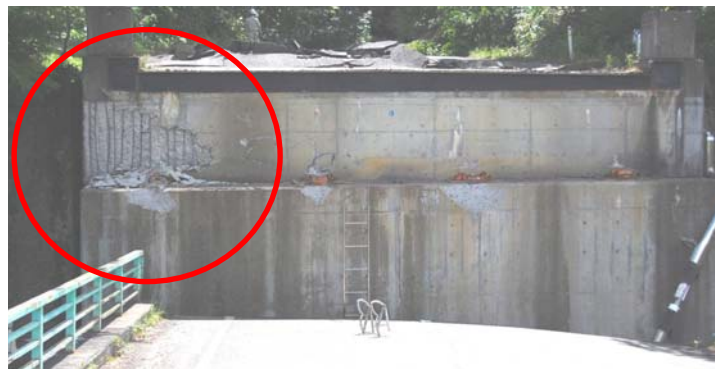
Figure 3.17 Pounding damage at the abutments in the transverse and longitudinal directions (KOERI, 2009; Kawashima, 2009)
