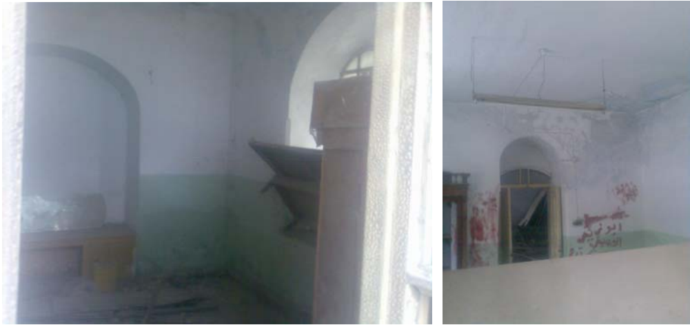
Figure 15.6: space 0.2, on the left looking south-west corner, on the right south-west corner
