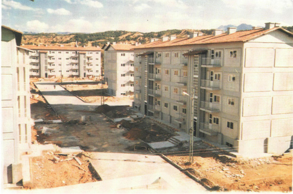
Figure 3. 5 Post-earthquake apartment buildings in Genç in Bingöl after 1971 earthquake.
