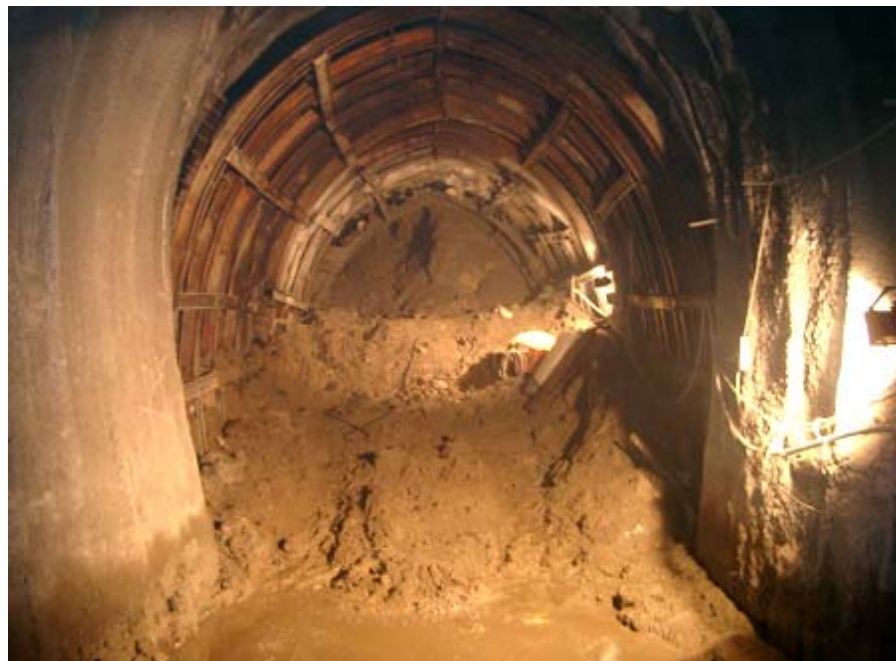
Figure 7-3 Huge collapse as a result of remarkable amount of convergence in squeezing ground condition in Malatya Railroad Tunnel
