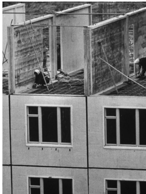
Figure 2.34. Construction of Khrushchevka “Central State Archive of the City of Moscow” (“TsGA Moskvi”)
