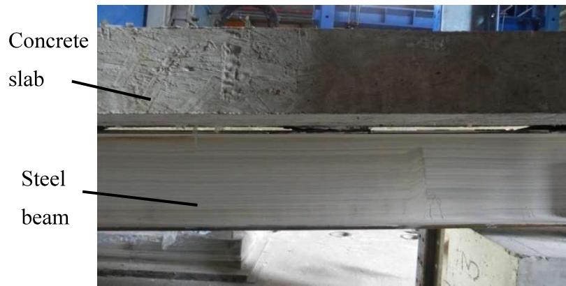
Figure 3.17. Separation between deck and steel at the end of test of Specimen-3
