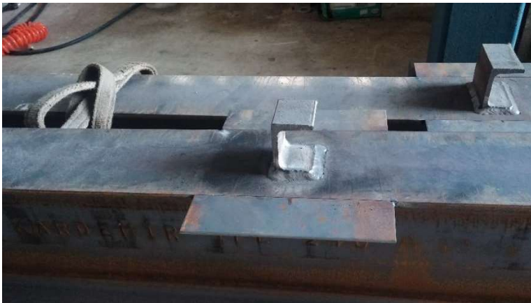
Figure 3.3. The channel shear connectors welded onto steel section with plates in two sides
