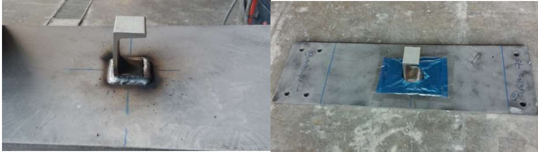
Figure 2.6. Channel shear connectors welded onto steel plate (a) The nylons covered at the bottom of shear pockets (b)
