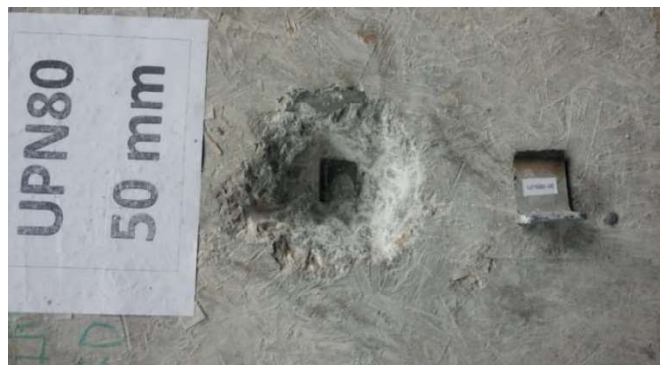
Figure 2.23. An example of concrete damage around channel shear connectors
