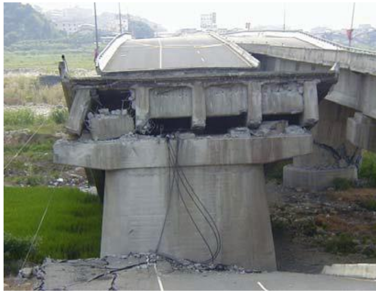
Figure 1.5. Wushi Bridge after Taiwan 1999 Earthquake (Chang et al., 2000)
