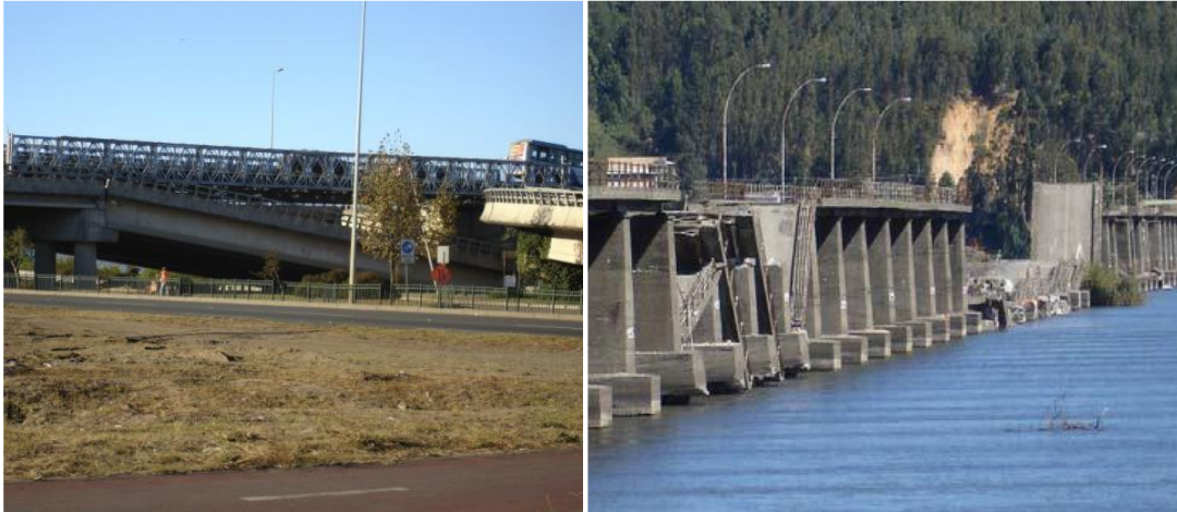
Figure 1.6. Unseated decks of Llacolen Bridge (on left) and Bio-Bio Bridge (on right) after Chile Earthquake 2010 (Escribano and Bhattacharya, 2011)
