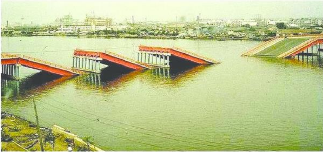
Figure 1.3. Collapse of the Showa Bridge after 1964 Niigata Earthquake (NISEE)
