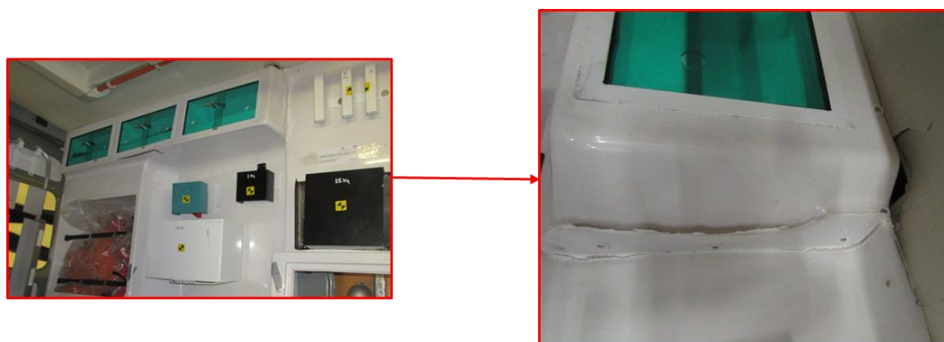
Figure 6.5. Second finding by post-test inspection
