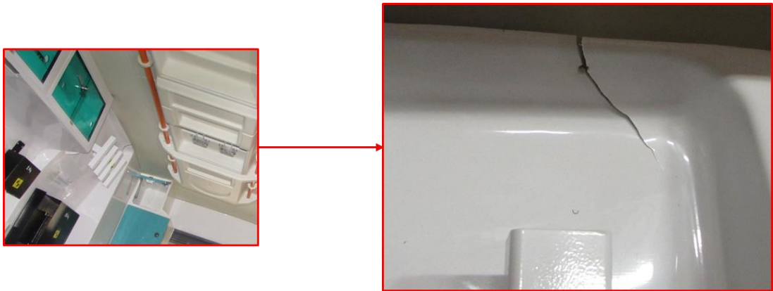
Figure 6.7. Fourth finding by post-test inspection
