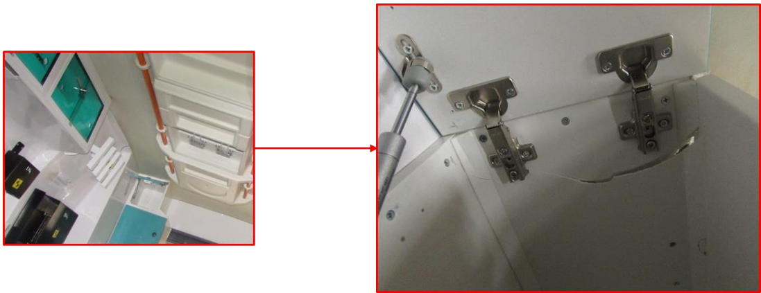
Figure 6.6. Third finding by post-test inspection
