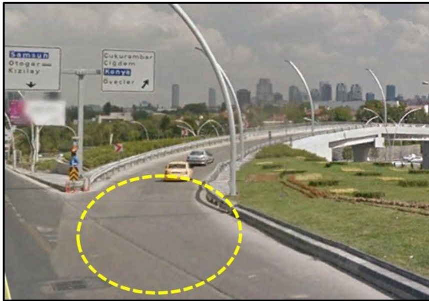
Figure 6.14. Absence of Delineation on Bridge Structure and Its Approach Roadway
