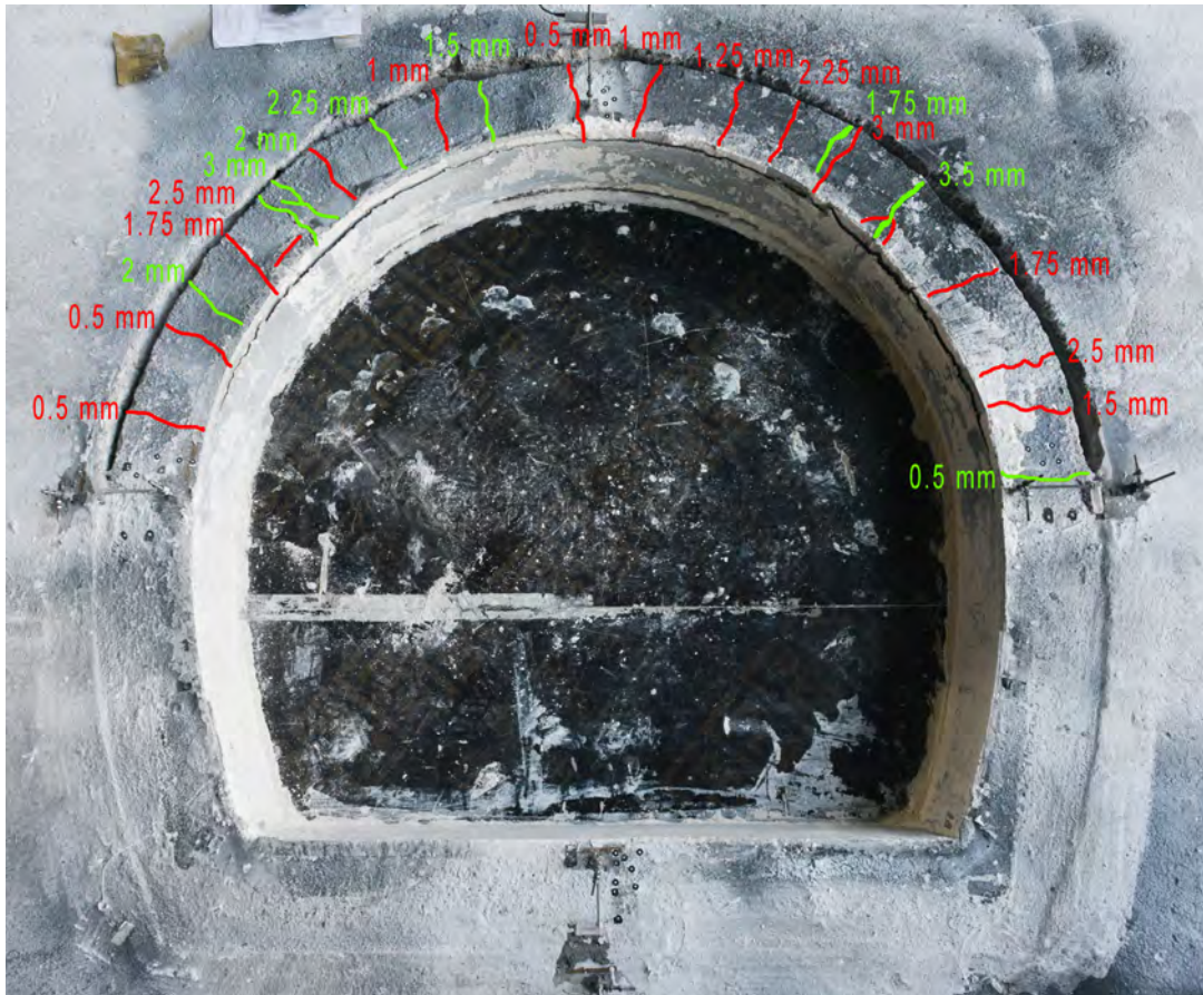
Figure 4.50: Crack map after HCIR experiment (cracks from previous experiment are marked with green)
