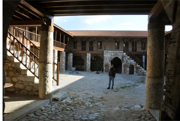
Figure 4.77. Çöllüoğlu Han before the restoration (top, middle) (Milas Municipality Archive), after the restoration (bottom) (Author, Dec, 2016).
