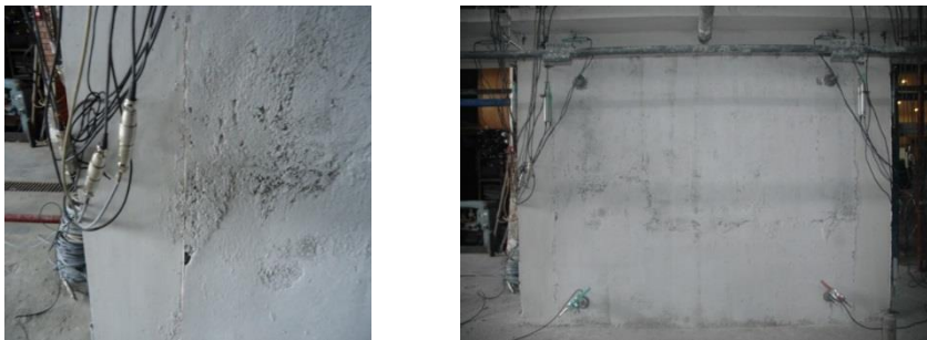
Figure 4.12 Observed damages related to D1 earthquake (strengthened frame)
