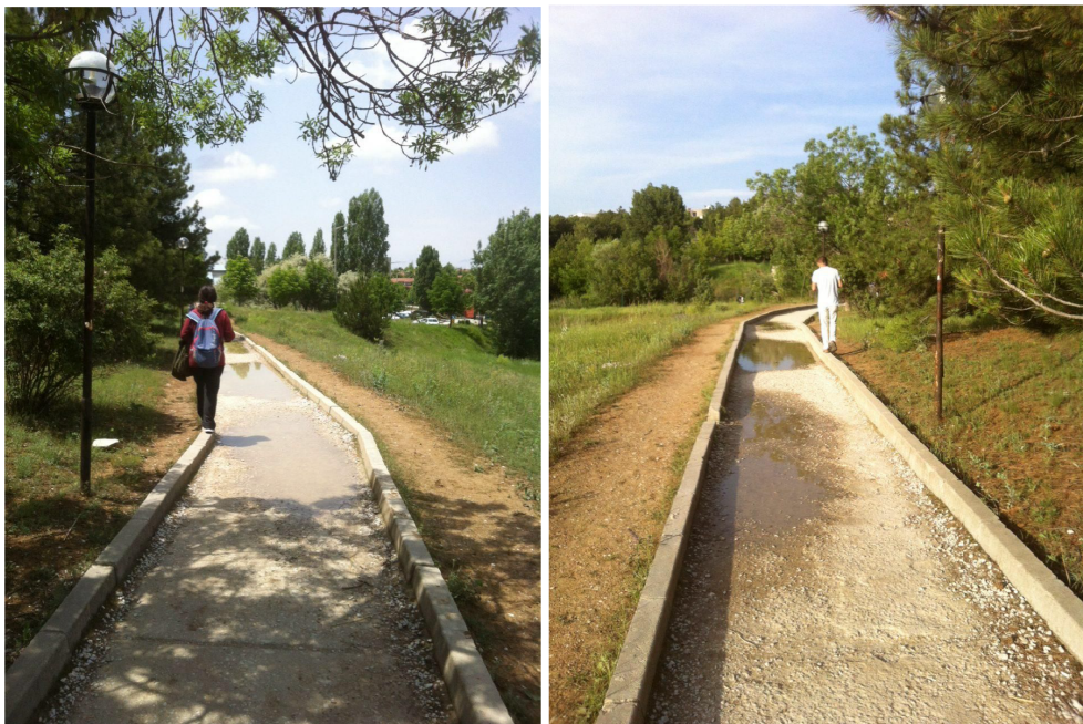
Figure 4.31: Poor condition of pavements. Picture is taken by one of the interviewees.
