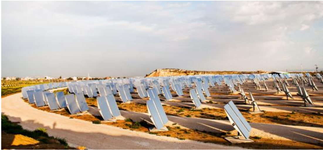
Figure 1 Installed CSP System in Mersin [4]
