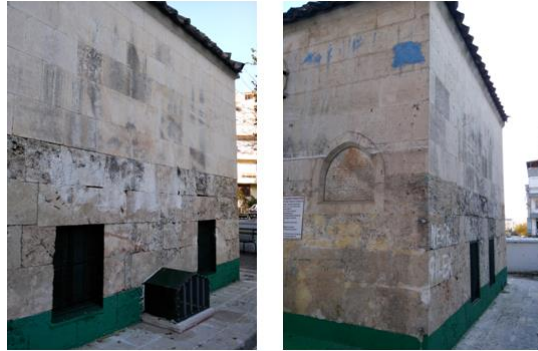
Figure 89 Southern Facade of the Şeyh Şüca Tomb in the Left and Western Facade of the Şeyh Şüca Tomb in the Right
