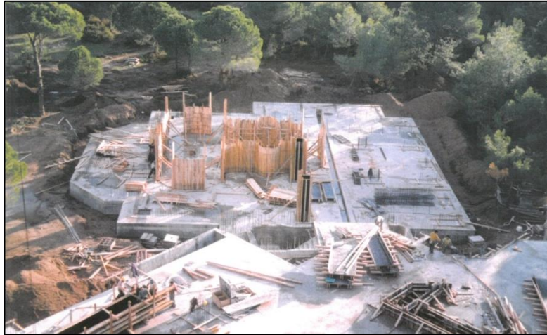
Figure 106 A photograph from construction period (archieve of Ministry of Culture and Tourism).
