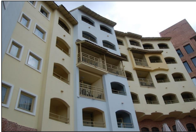
Figure 64 Various opening configurations on the same facade (taken by the author, December 2013).
