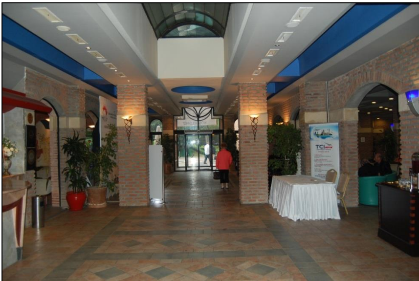
Figure 52 The toplight over the lobby is covered with a plastic material (taken by the author, December 2013).
