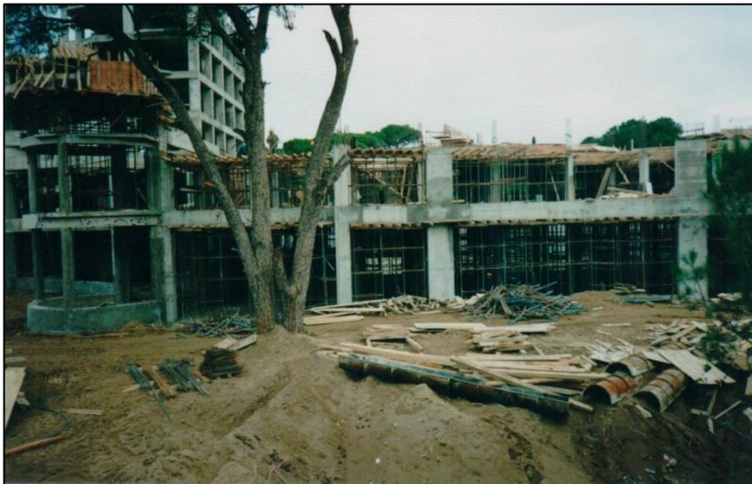
Figure 71 A photograph from construction period (archieve of Ministry of Culture and Tourism).
