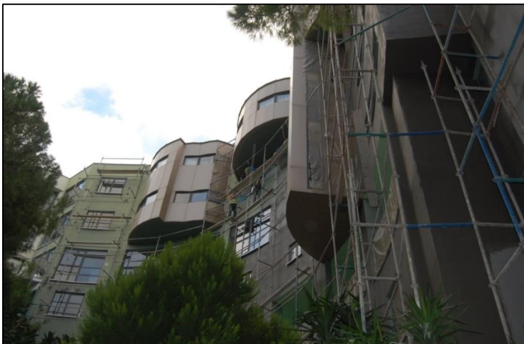
Figure 103 The construction work to install thermal insulation (taken by the author, December 2013).
