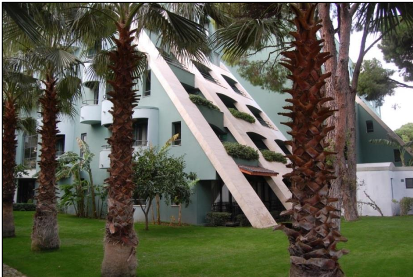
Figure 102 The parapet walls near the balconies of the P Block (taken by the author, December 2013).
