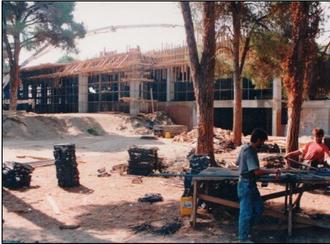
Figure 31 A photograph from construction period (archieve of Ministry of Culture and Tourism).
