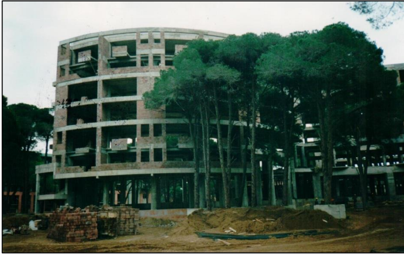
Figure 70 A photograph from construction period (archieve of Ministry of Culture and Tourism).
