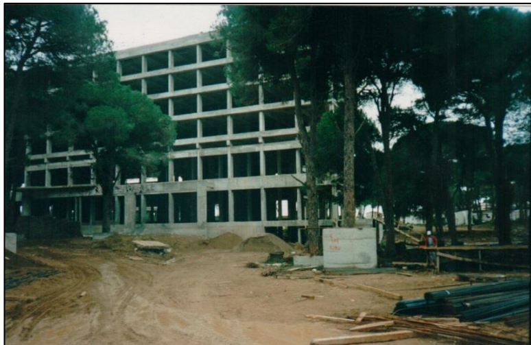
Figure 30 A photograph from construction period (archive of Ministry of Culture and Tourism).
