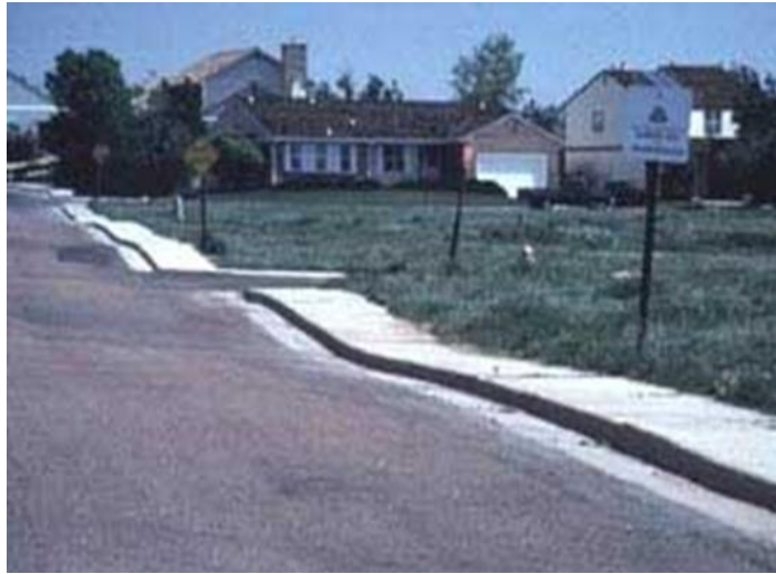
Figure 1.3 A view of road undergoing swelling
