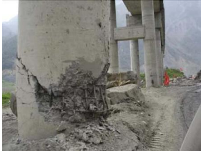
Figure 3.2 Baihua Bridge After 2008 Wenchuan Earthquake (Adopted from Han et al., 2009)
