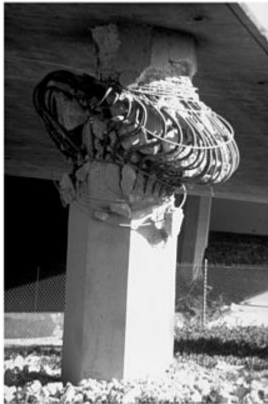
Figure 3.1 Concrete Bridge Columns After the 1994 Northridge Earthquake, California (Highway 118/Bull Creek Bridge) (Adopted from NISEE e-Library, 1994)
