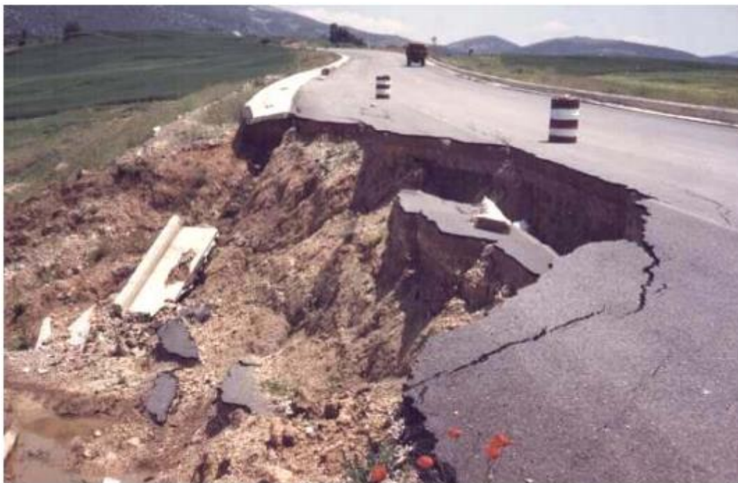
Figure 3.4 Road Embankment Failure Caused by Lateral Slumping During the 1995 Kozani Earthquake, Greece (Adopted from SYNER-G Project 244061, 2011)
