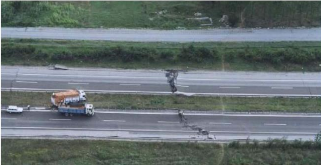
Figure 3.3 Damage to Highway Caused by Fault Rupture During the 1999 Kocaeli Earthquake, Turkey (Adopted from SYNER-G Project 244061, 2011)
