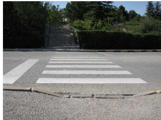
Figure 6: Discontinuity of the curb ramp on the most commonly used pedestrian crosswalk
