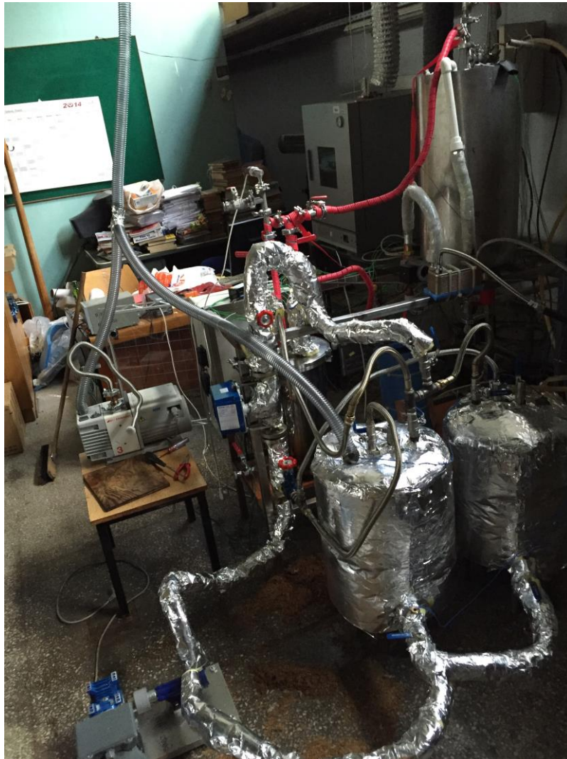
Figure 4.27 The insulated and installed HTF tanks and HTF loop
