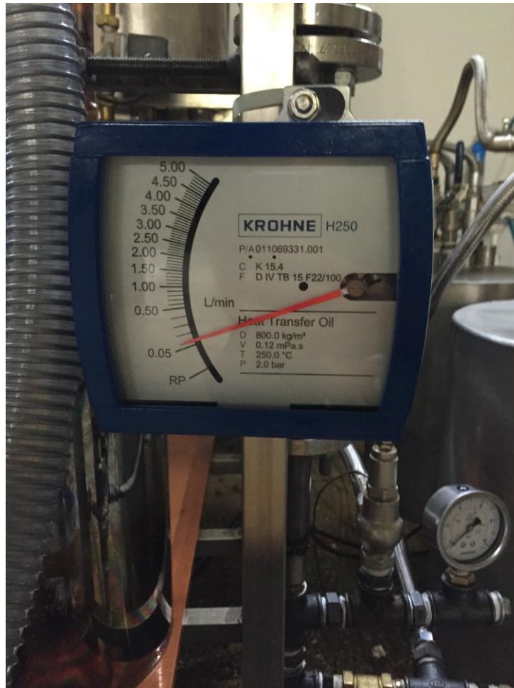
Figure 4.30 Photograph of the HTF flow meter
