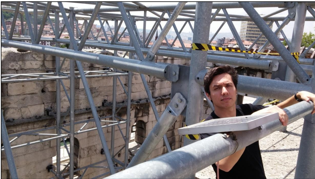
Figure A.10: Windows on the southeastern wall and the solar panel of SHM system
