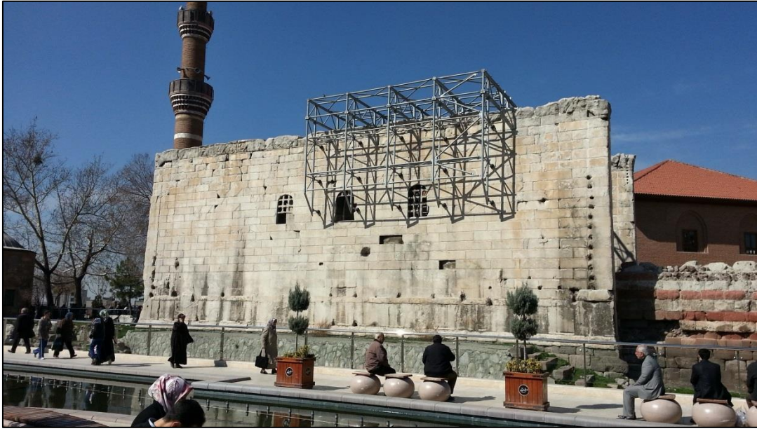
Figure A.2: General view from the eastern vantage point, holes are visible all around the wall
