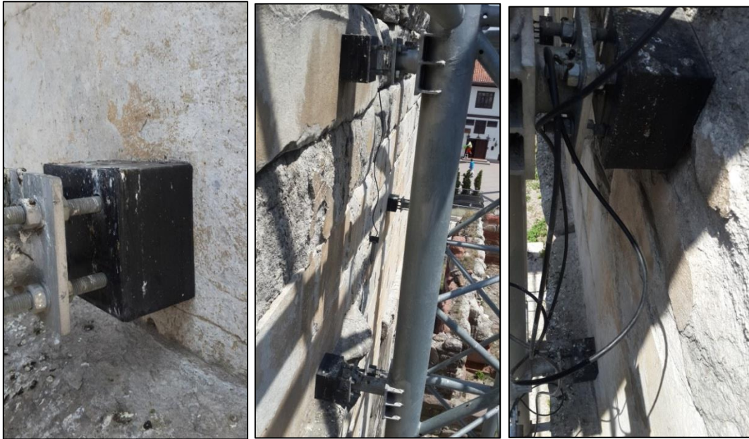
Figure 2.26: Rubber pads in contact with wall surface
