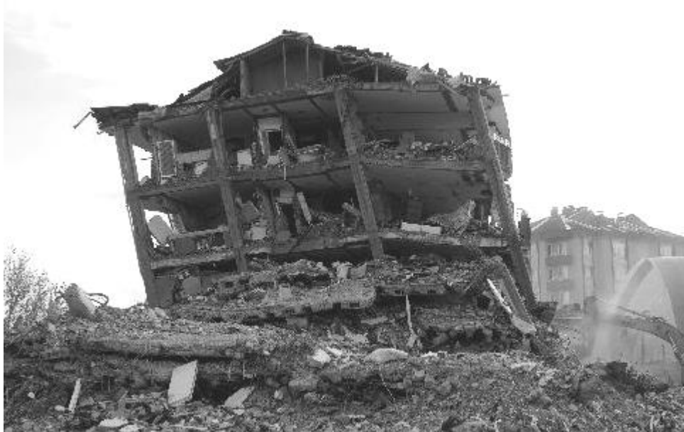
Figure 1.2. A collapsed Asmolen building in Erciş, 2011 Van Earthquake (Dönmez, 2013)
