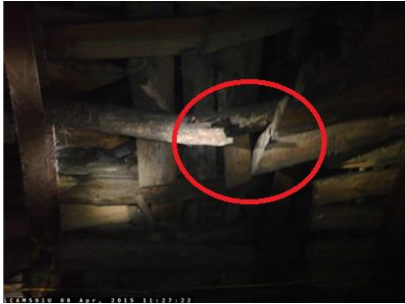
Figure 4.3 An Example of an Inadequate Support in the Study Area
