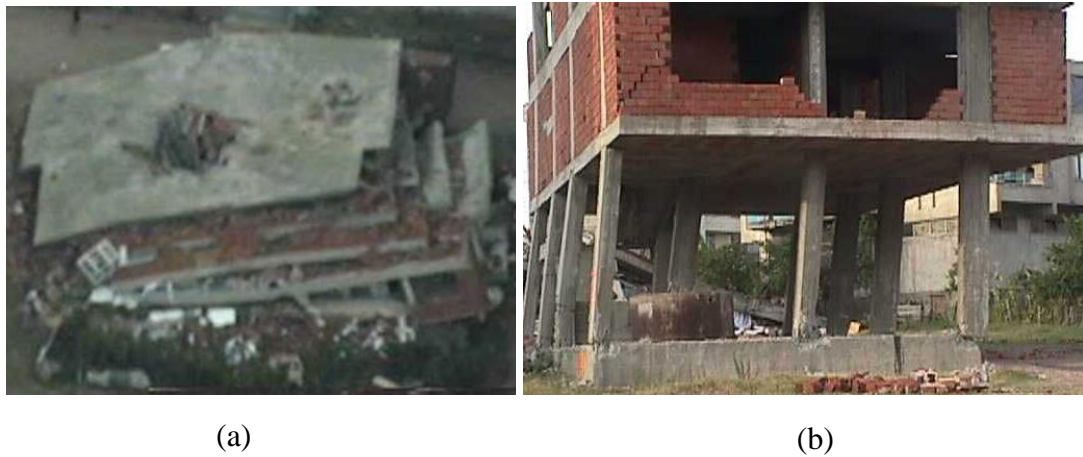
Figure 3.1 Examples of the story mechanism induced by the hinge plasticization at the column tips of RC MRF buildings
