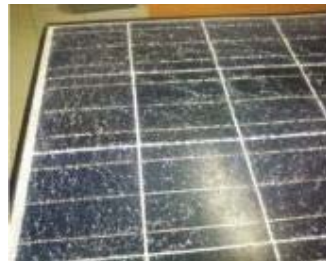
Figure 1-21 Severely broken glass on a polycrystalline PV module [59]
