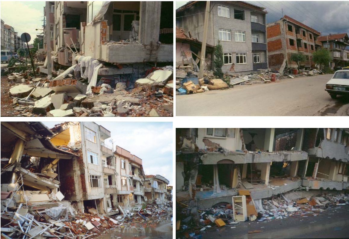
Figure 3.9 Ground floor destruction due to high ductility demands (photos courtesy of METU-DMC)
