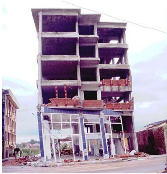
Figure 3.8 Failure due to the soft story irregularity (photo courtesy of METU-DMC)
