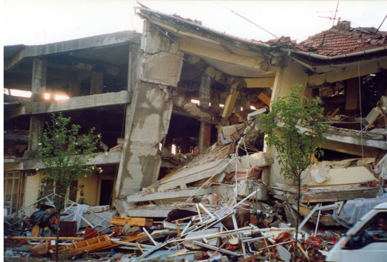
Figure 3.12 Anchorage problems at beam-column connections (photo courtesy of METU-DMC)
