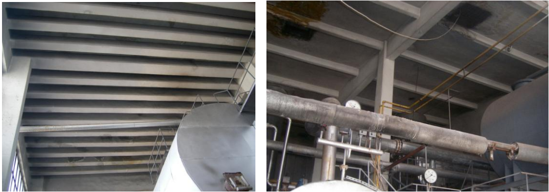
Figure 77. The photographs showing the differences on the structural systems of the original and additional building (Source: Author)
