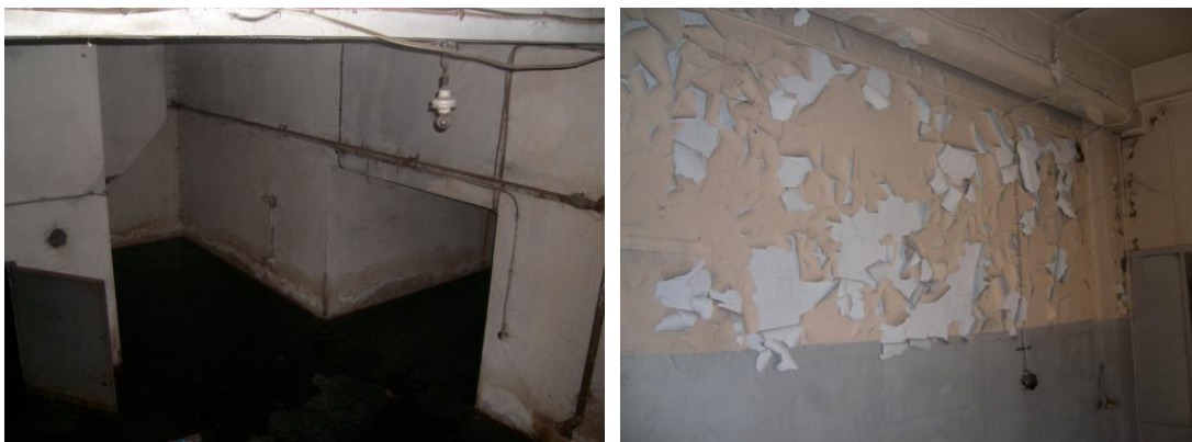
Figure 57. The water accumulation on basement floor due to drainage problems and the deformations on painted surface. (Source: Author, 2012)
