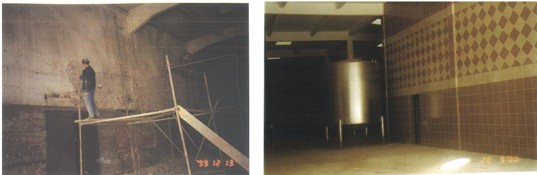
Figure 73. The inner walls of the beer filling building before and after the repairs made in 2001 (Source: TTA Archive)
