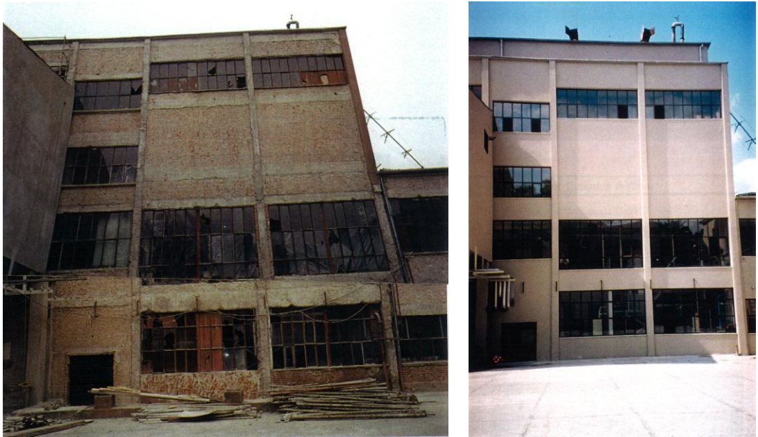
Figure 83. Photographs of the south façade of the boiling and fermentation building which were taken before (left) and after (right) the repairing in 2001 (Sources: TTA Archive)
