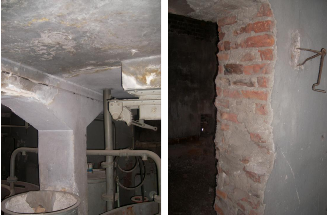
Figure 47. The column, beam and brick masonry structure of the production part in the old factory building (Source: Author, 2012)
