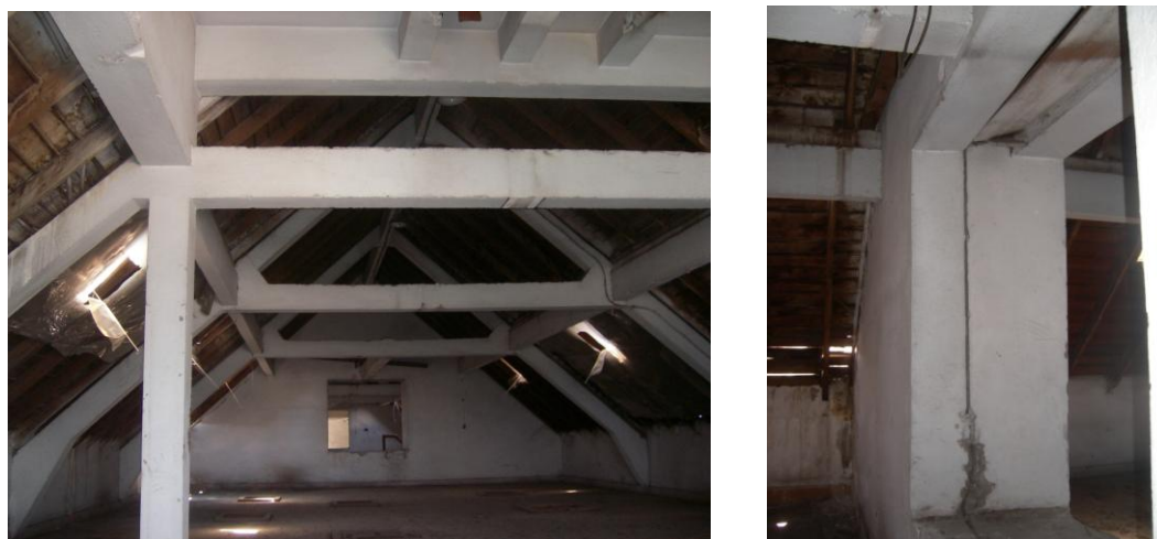
Figure 56. Combination of reinforced concrete and timber construction system on roof floor (left) and the dilatation showing the place of 1947 dated addition (right) (Source: Author)
