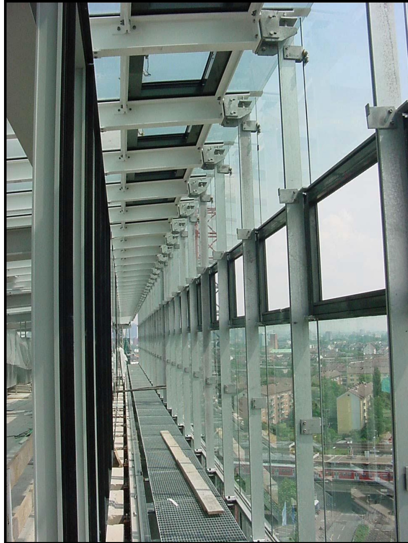
Figure 2.24. The Cavity of The Double Skin Facade Prisma House, Office Building, Frankfurt, Germany, 2001 (Source: Bayram, A., 2003)
