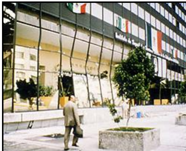
Figure 2.43. Glass Damage in Mexico City Earthquake, 1985. (Source:Arnold,2009)
