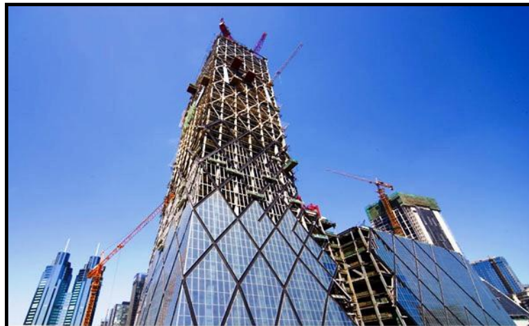
Figure B.2. The View from The Construction Stage of The Building ( www.janghogroup.com ,2012)
