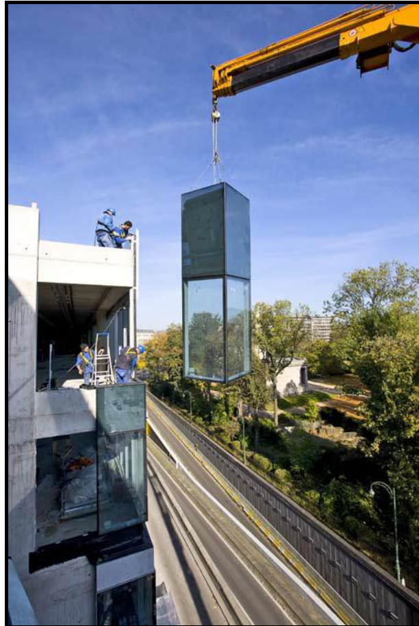
Figure 2.27. The Installation of Panel Curtain Wall System from The Exterior of Building (Source: Metal Yapı, 2012)
