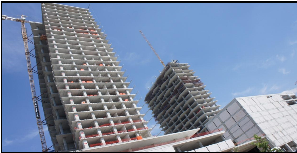
Figure B.10. The Photo from The Construction Stage of The Building (Source:www.nextlevel.com,2012)
