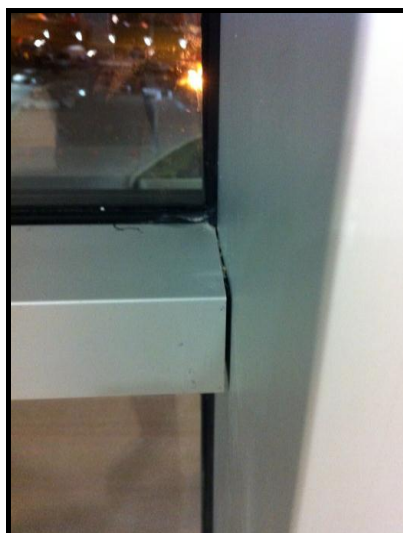
Figure 2.44. The Fault In The Horizontal and Vertical Connection of Aluminium Members. (Source:Individual Archive of The Author, 2012)
