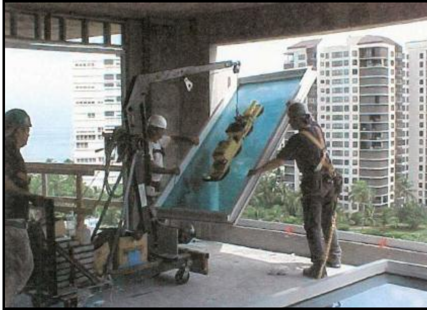
Figure 2.10. The Installation of Panels With The Help of Suction Cups, (Source: www.bcindustries.com)
