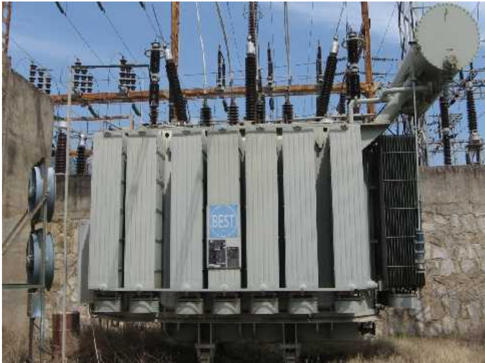
Figure 4.9: 50 (62.5) MVA Power Transformer
