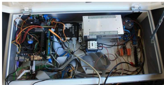
Figure 3-24: Computer box with main control units (left) and regulators (right)
