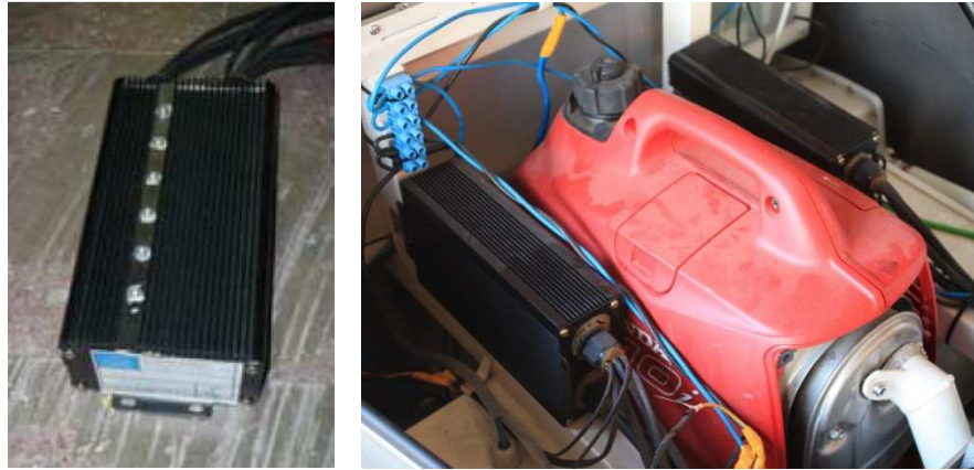
Figure 3-18: Hub motor driver (left). Drivers located next to the generator (right)
