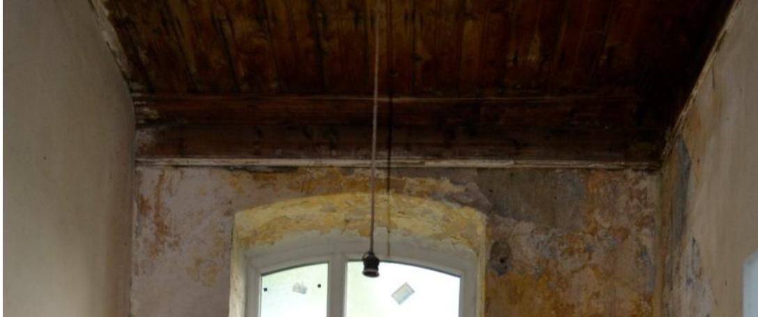
Figure 25: Additional partition wall on left, Tarabya R.İ.O. Wooden works on meeting point of ceiling and wall does not continue on left side, where additional wall meets ceiling. (Author, June 2011).
