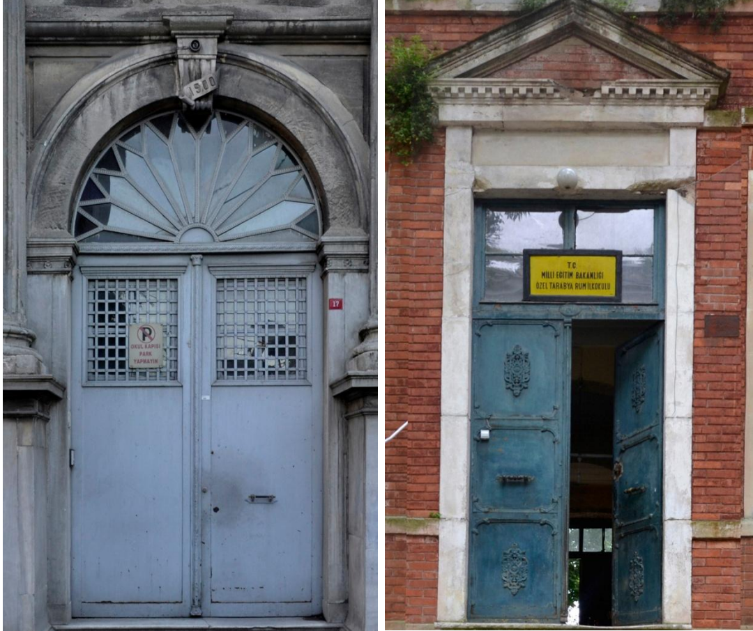
Figure 17: a) Entrance door of Maraşlı R.İ.O.; spanned with arch, different than interior doors which are spanned with lintel. b) Entrance door of Tarabya R.İ.O.; made of metal, different than timber framed interior doors.
