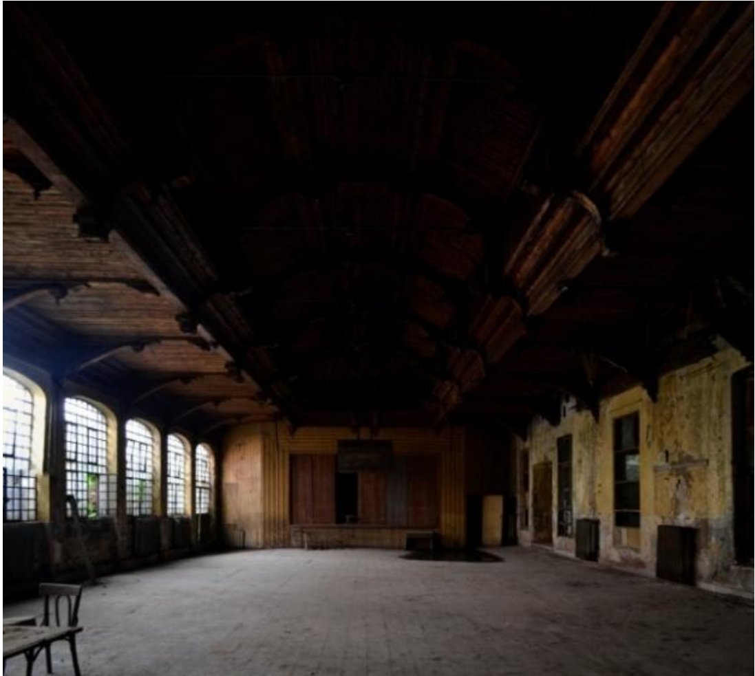
Figure 12: Hall of ceremonies / gymnastic saloon of Merkez R.İ.O.L. Highly detailed timber framed construction of roofing is a rare example that the school building features (Author, June 2011).
