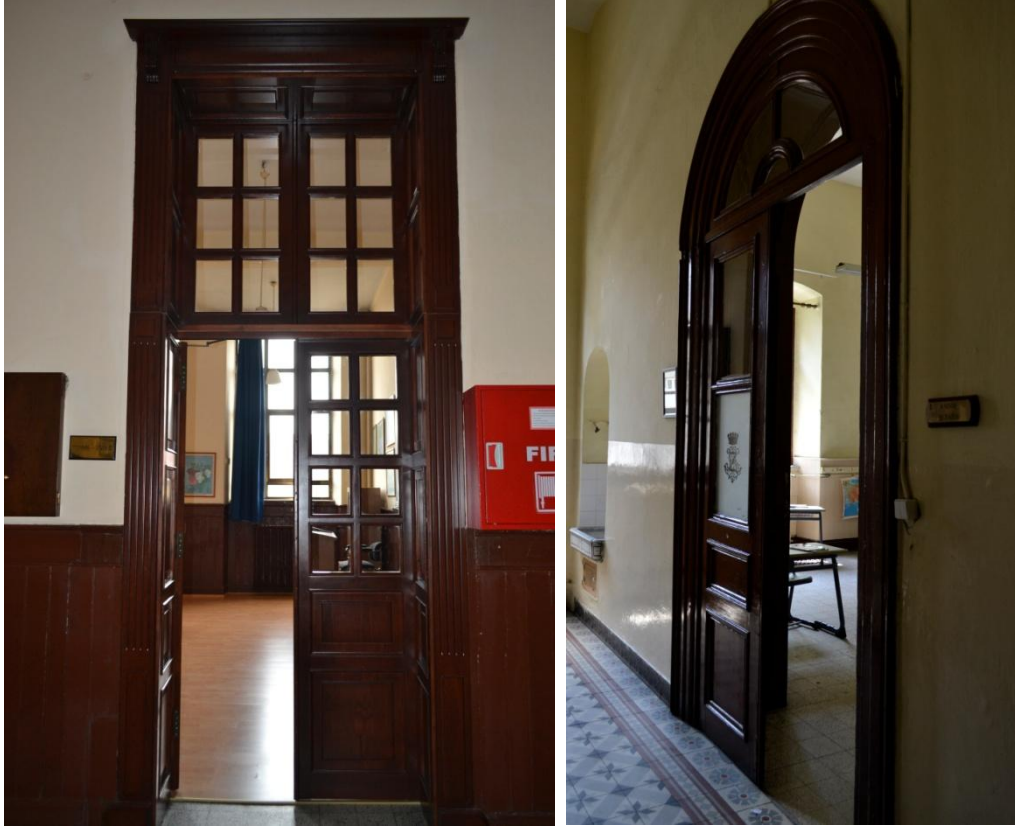
Figure 16: a) Door opening of a classroom in Zoğrafyon R.L.İ.O., which is spanned with lintel. b) Door opening of a classroom in Zapyon R.İ.O.L., which is spanned with a central arch. (Author, June 2011).
