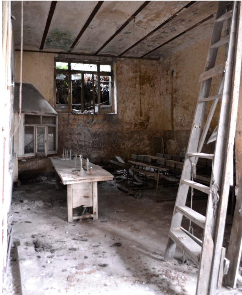
Figure 21: View of a laboratory space, Merkez R.İ.O.L. The broken window frames causes more deterioration inside.
