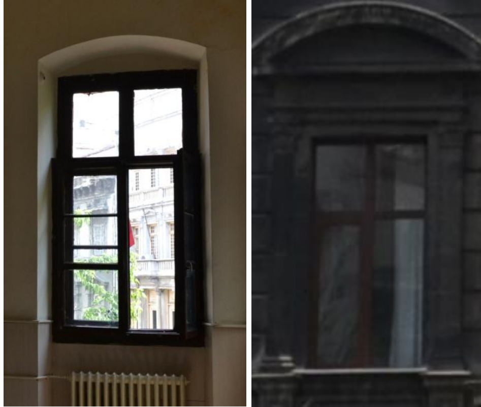
Figure 15: a) Interior view of a window opening, Zapyon R.İ.O.L. It is seen that the opening is spanned with a segmental arch. b) Exterior view of the window opening, Zapyon R.İ.O.L. From outside the opening is perceived to be spanned with a lintel (Author, June 2011).
