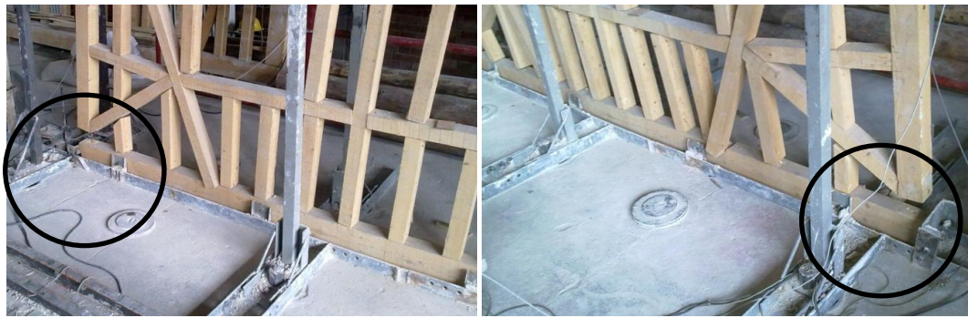
Figure 149: Permanent connection failures of the Frame#8 after the test
