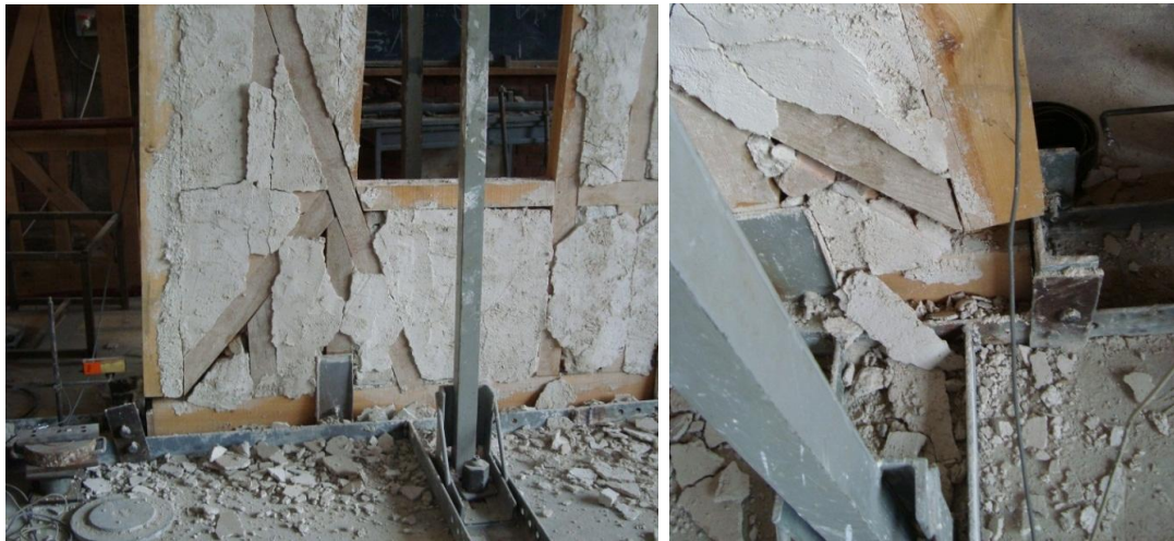
Figure 112: Examples to connection failure
