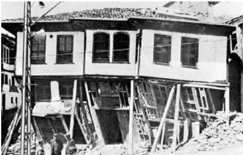
Figure 37: A timber-framed building damaged due to the weakening of the ground floor by enlargement of the openings (after Şahin-Güçhan, 2007a)
