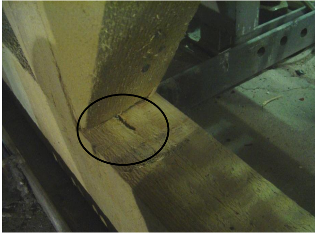
Figure 81: Trace of the slipped nail
