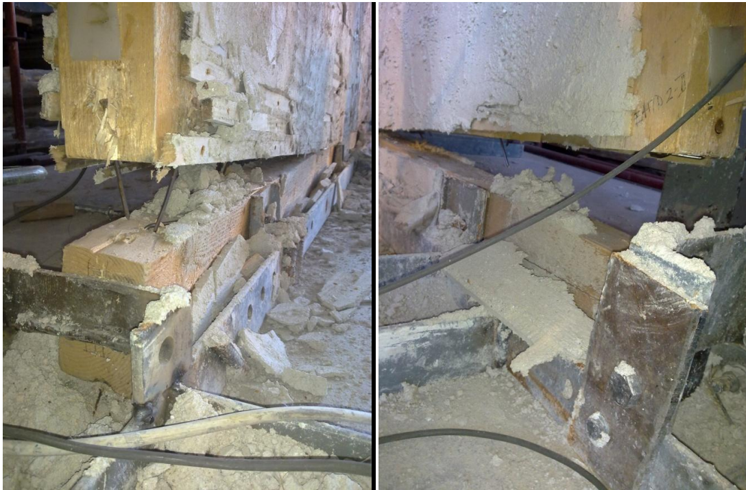
Figure 156: Examples to connection failures observed during the testing of Frame#8 with bağdadi covering
