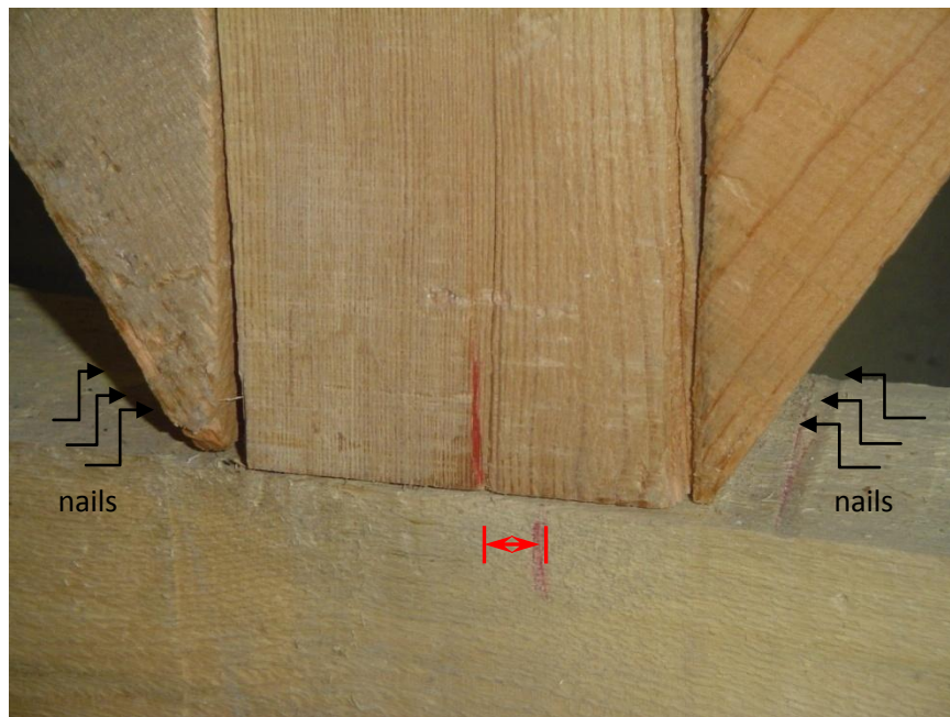
Figure 93: Displacement occurred at the middlemost upright element during Test#3
