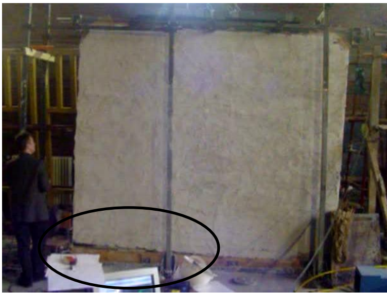
Figure 99: Dilatation at the frame bottom
