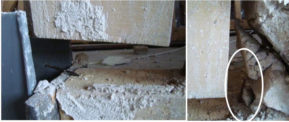
Figure 144: Examples to buckled nails
