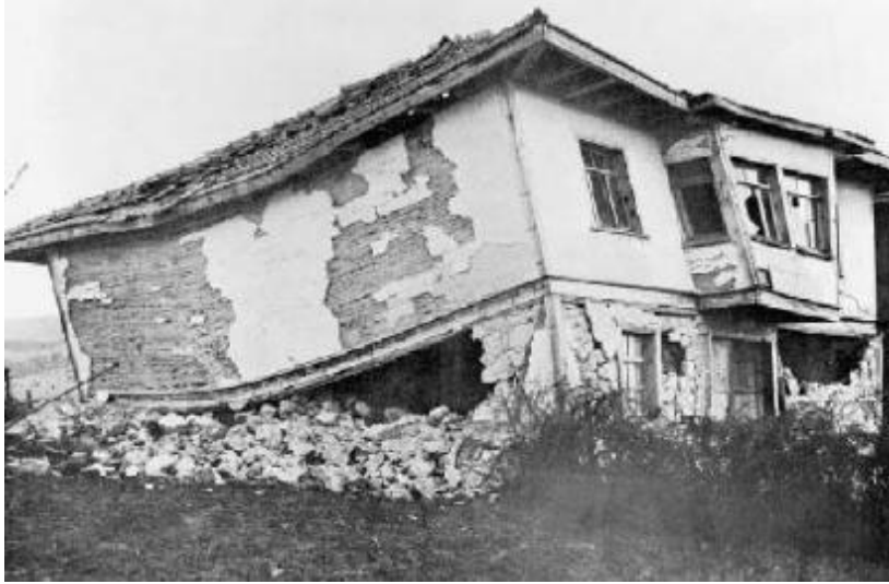
Figure 36: An example showing the destroyed masonry ground floor in Iğdiş Village after 1970 Gediz Earthquake (after Şahin-Güçhan, 2007a)
