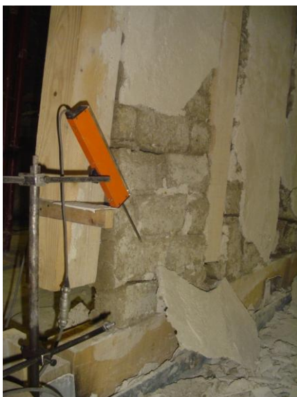
Figure 88: An example to connection failures
