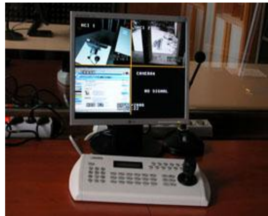
Picture 5: The control room
