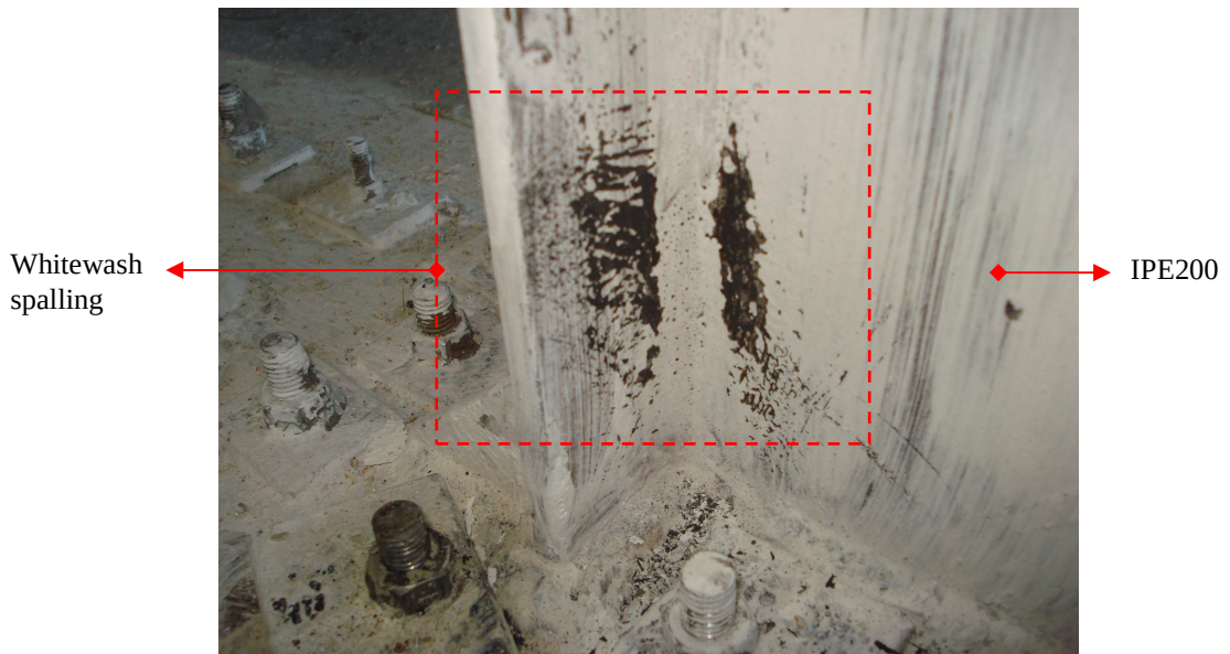
Figure 3.64 Yielding of steel column C3
