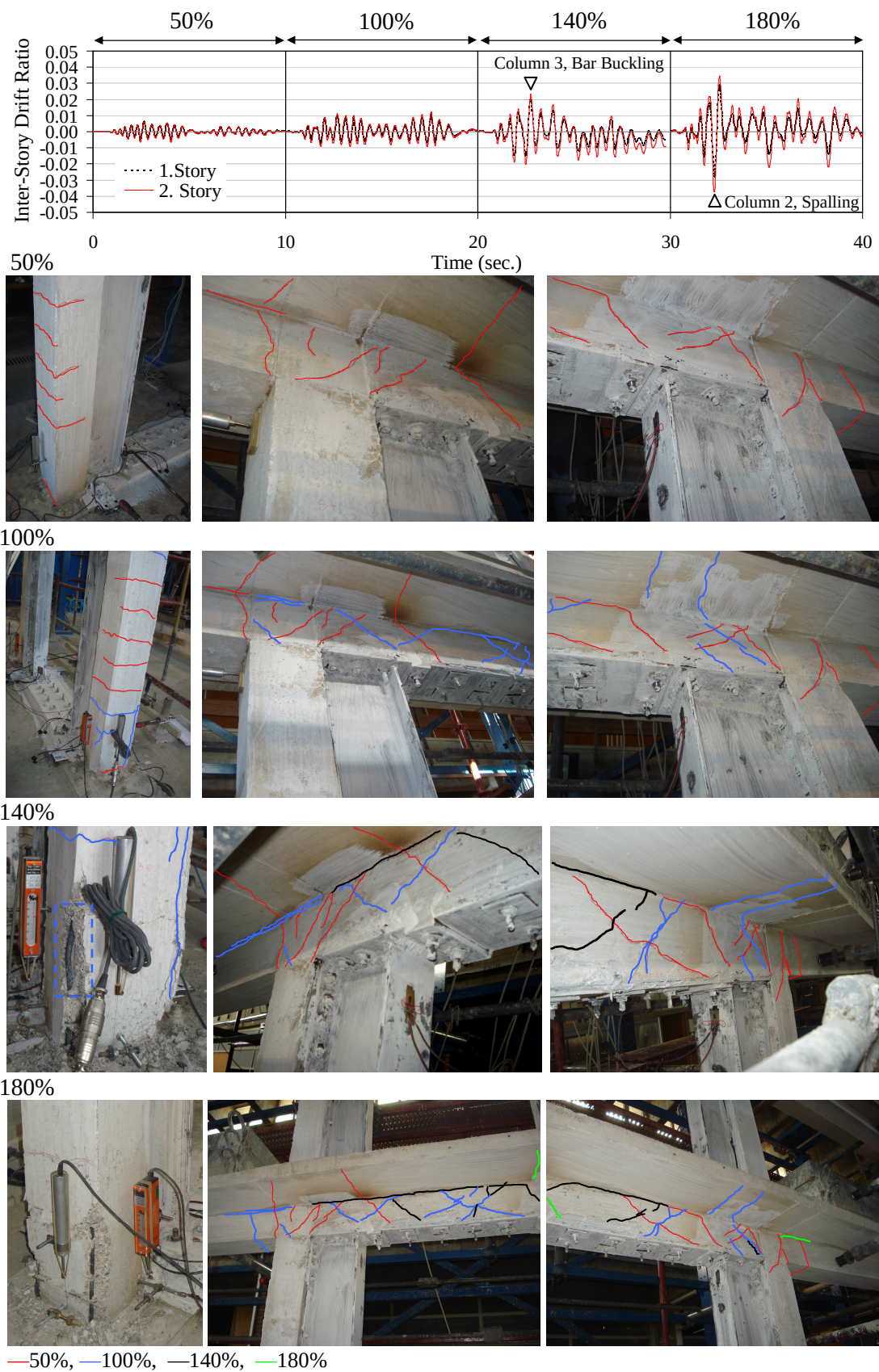
Figure 3.63 Physical damage of the ISF
