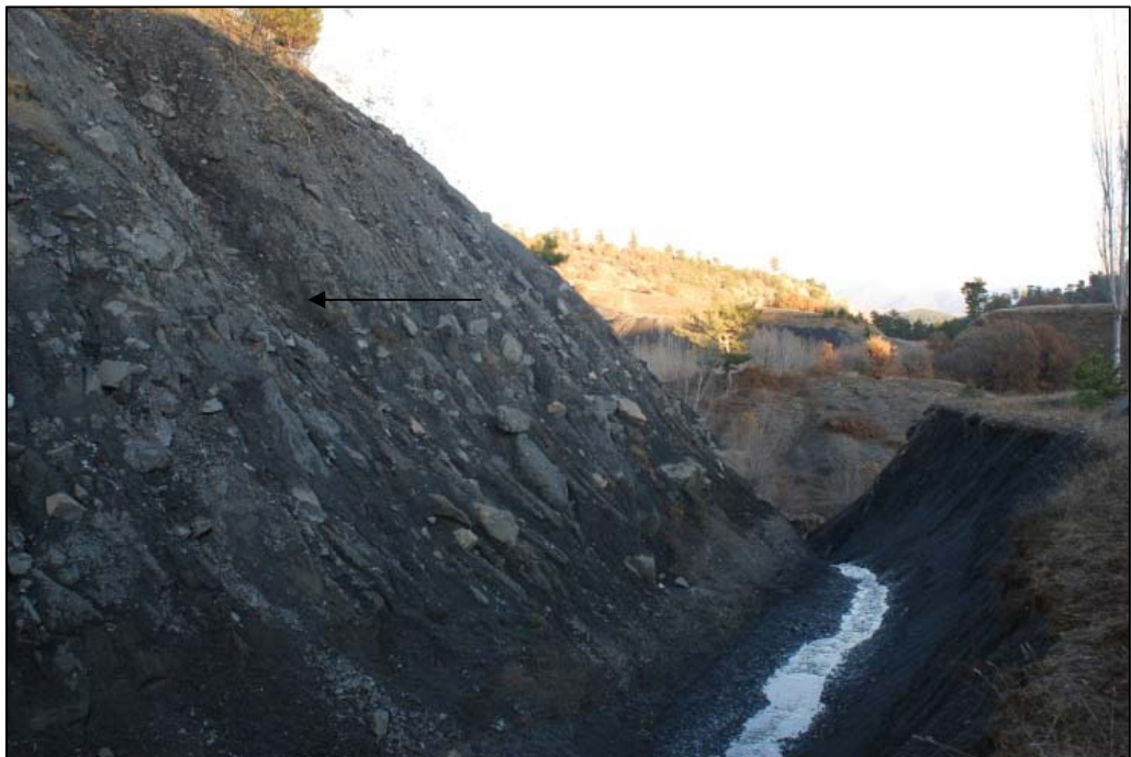
Figure 9 A view from slope of the dump site showing erosional processes (rill formation)
