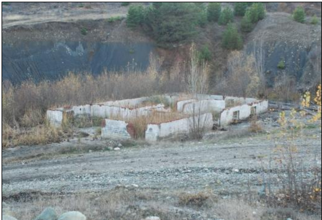
Figure 11 Flooded coal storage building
