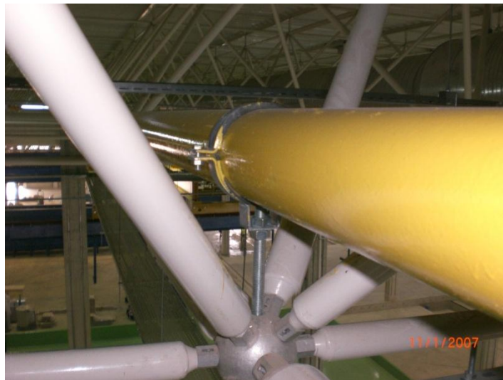
Figure – 3: A gas pipe passing along the roof
