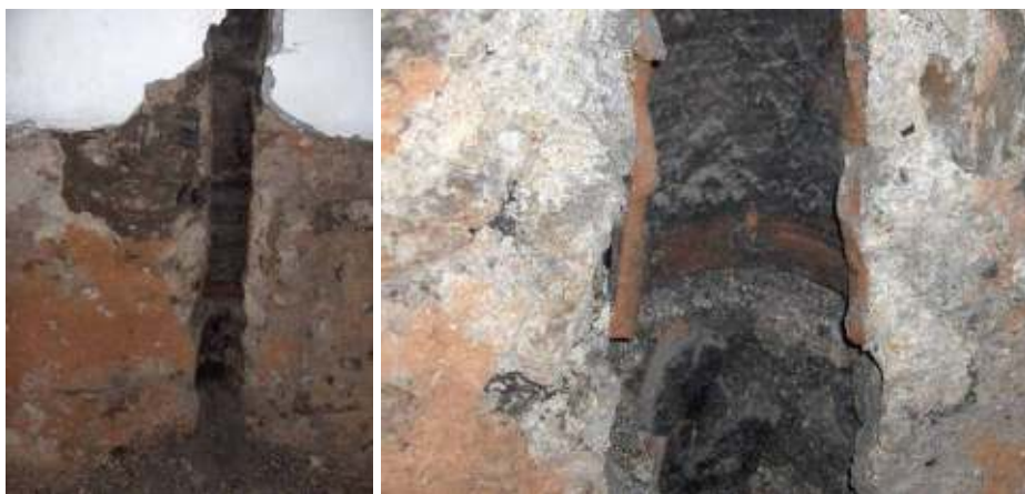
Figure 2.5 Views of terracotta draft chimneys ( tüteklik ) rising inside the wall up to the roof in Yıldırım Beyazıt Hamamı in Mudurnu, Bolu (Source: Archives of Gülşen Dişli ).
