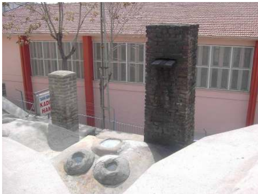
Figure 3.6 View of two draft chimneys; one out of use (on the left) and one with a damper mechanism to open and close the top (on the right) on the roof of Şengül Hamamı (Source: Archives of Author)
