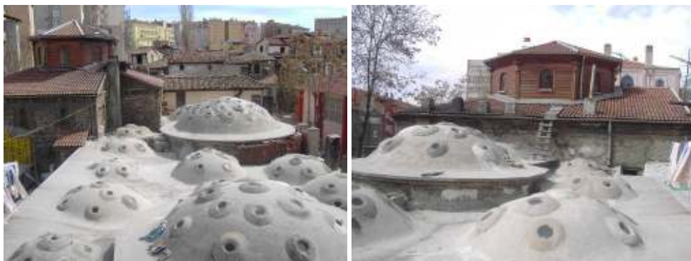
Figure 3.8 Views of Şengül Hamamı's roof covered by an 8 cm-thick mesh-reinforced concrete layer (Source: Archives of the Author)
