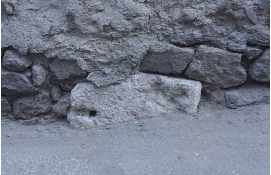
Figure 12: Another architectural member re-used for the wall construction at Atpazarı Sokak (Photo: Emre Kaytan).
