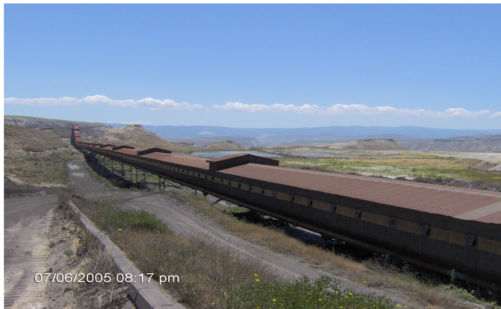
Figure 2.8 Closed conveyor belts
