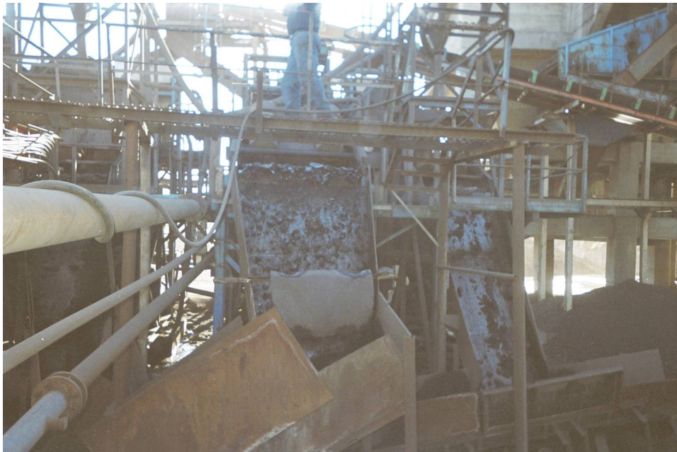
Figure 2.4 Coal washing unit
