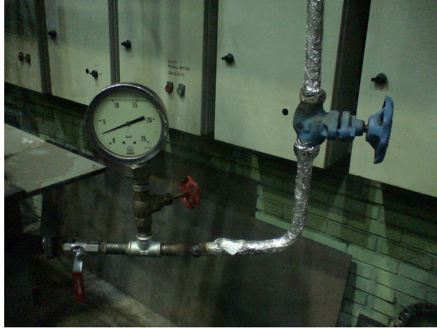
Figure 4.29 View of the Pressure Reading System.
