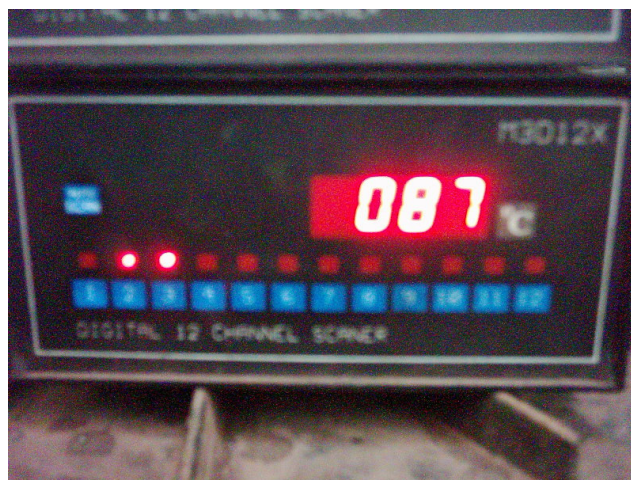
Figure 4.30 View of the Temperature Reading System M3D12x.
