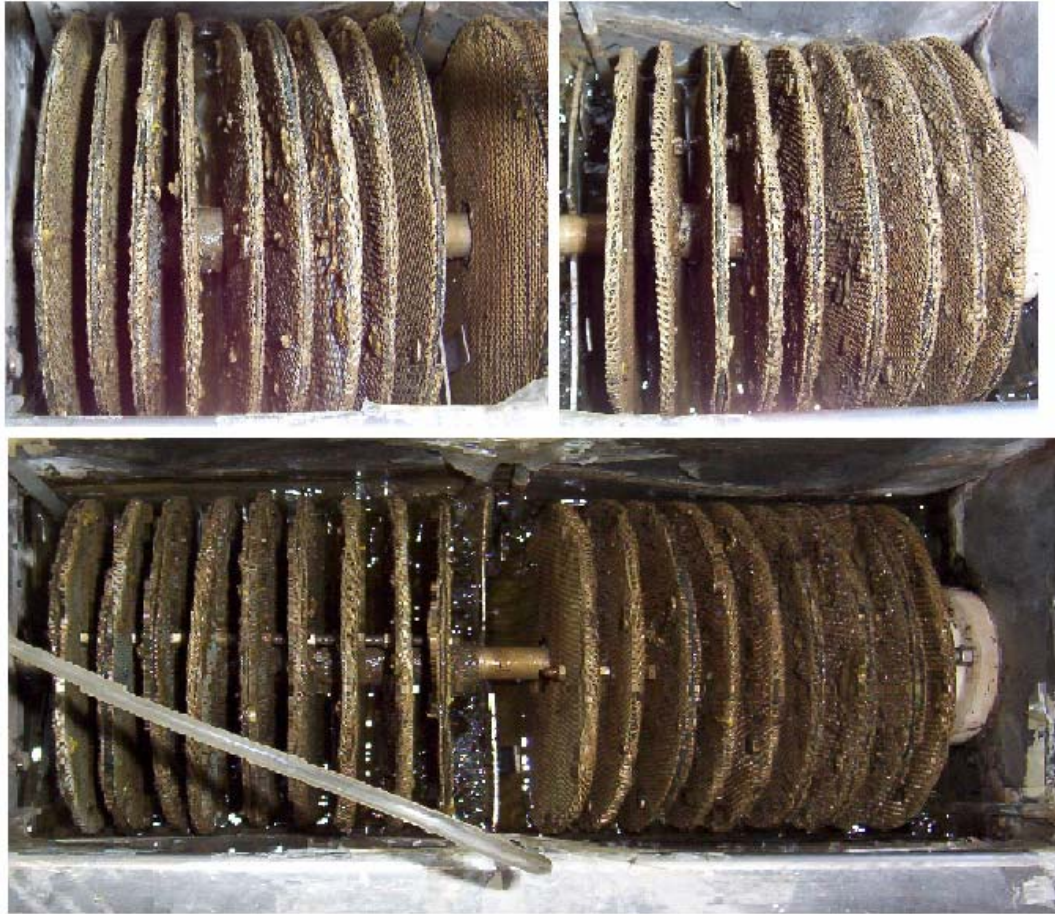
Figure 3.59. RBC discs after additional aeration
