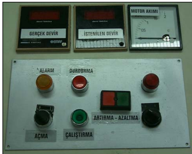
Figure 50 Old Fan Driver RPM Controller
